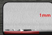
Edge band not glued properly
